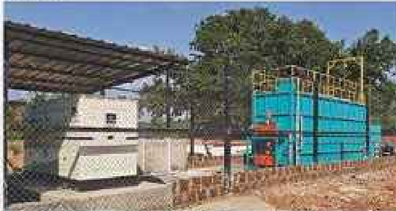
100 KLD Sewage Treatment Plant at fisheries Jetty, Cutbona, Salcete - Goa.
