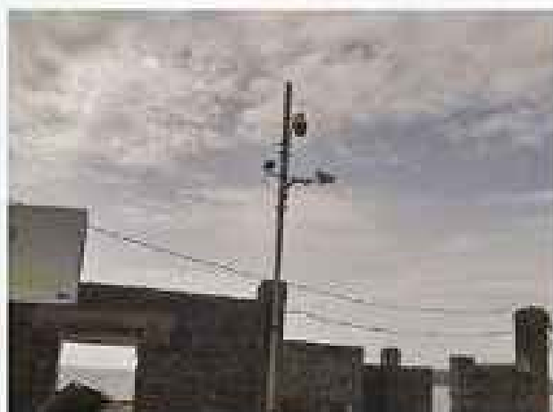
CCTV installed at Chapora Jetty
