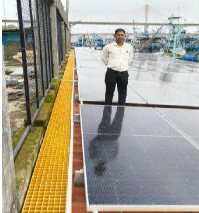
Newly installed Solar panel at Malim
