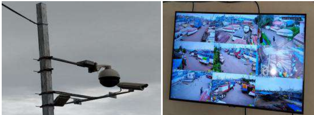
CCTV surveillance system at Cutbona Jetty
