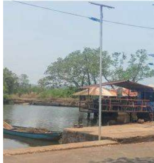
Solar lights installed at Amona – Bicholim
